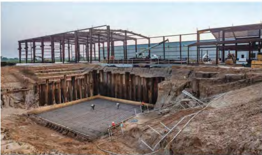
Seanic's in-ground tank measures 50ft x 50ft x 30ft deep.
