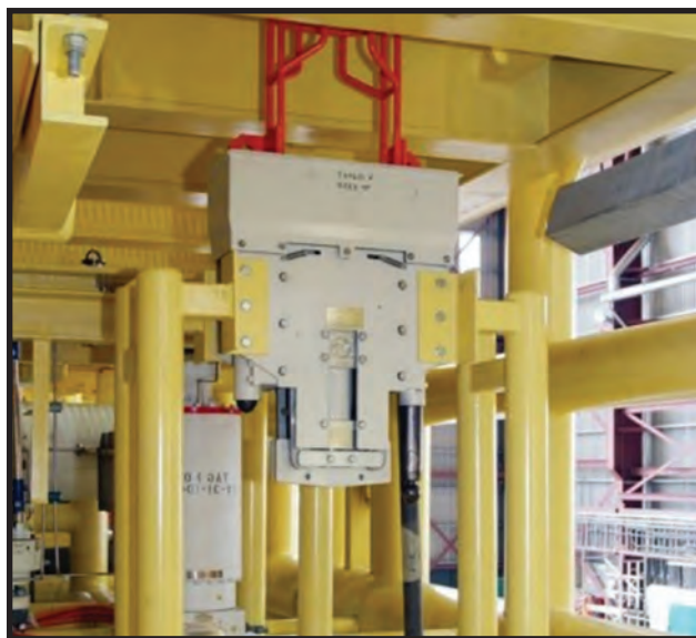
Figure 1: SECC's connector installed on a manifold. Images from SECC.
