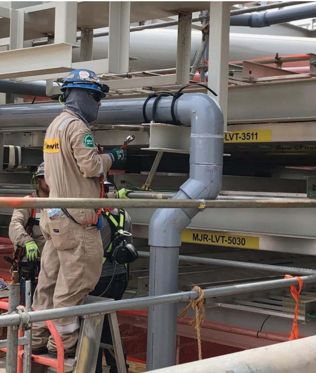
Field installation of the RedLineIPS SmartPad System, showcasing quick and efficient setup without the need for welding or epoxy.
